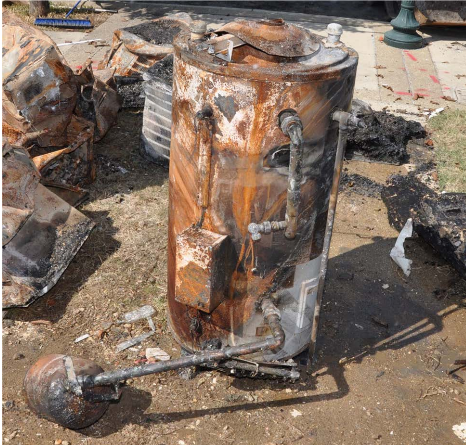
Figure 14. Hot water heater at the accident scene after the explosion. (Photograph provided by ATF.)
