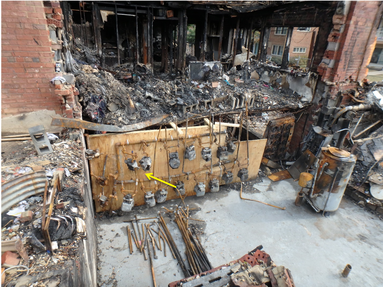
Figure 6. Building 8701 after debris removal and ATF reconstruction. The first two gas meters (designated with a yellow arrow) show substantially more heat/fire damage than other meters. (Photograph provided by ATF.)
